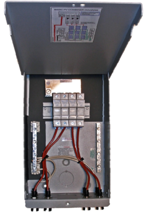
MNPV4 Factory wiring
